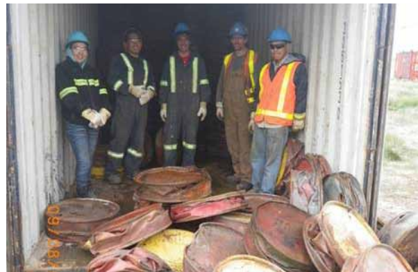
Above is the cleanup crew preparing some of the scrap metal to be shipped south.
