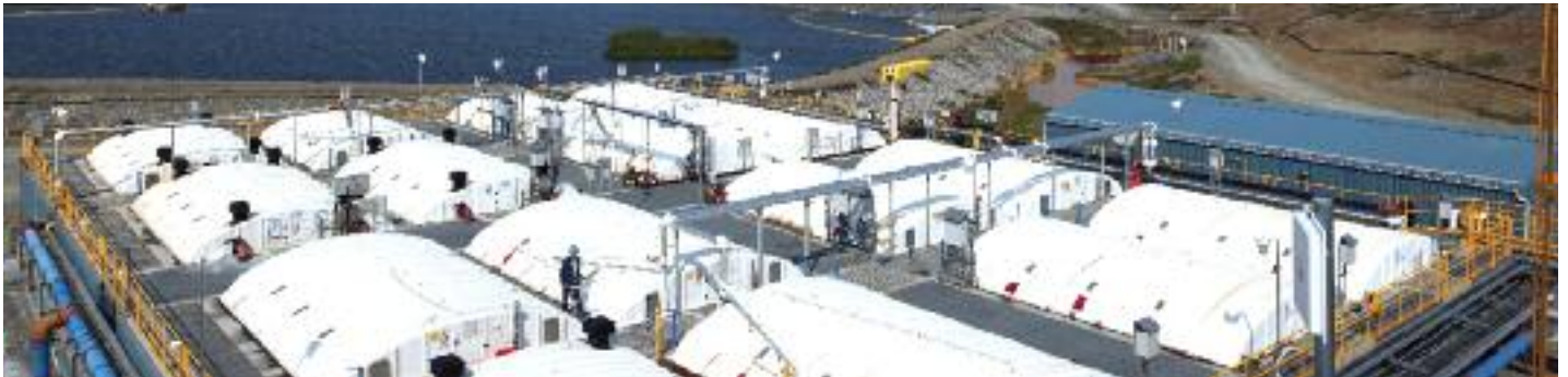
Process waste water treatment plant at the LaRonde mine
