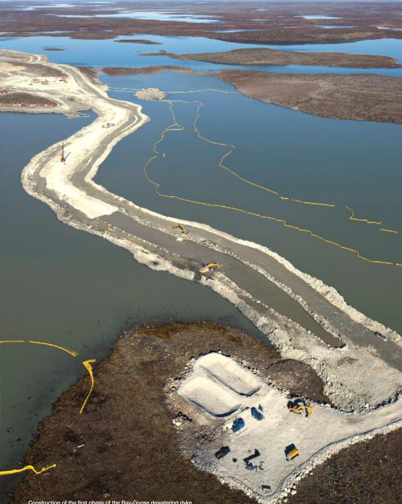
Construction of the first phase of the Bay-Goose dewatering dyke at the Meadowbank mine – Summer of 2009
